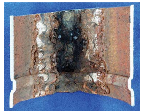
Figure 6. Pipe from dry FPS showing an air-water interface where a puddle had been. Note the discrete deposits and severe under-deposit pitting in this area.
